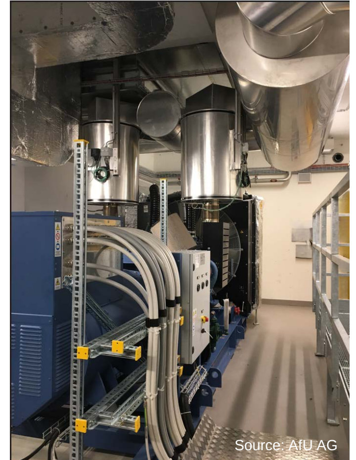
Emergency generator: 1500 kVA, 3.0\text{ MW}_{\text{th}} equipped with 2 DPF and a silencer
